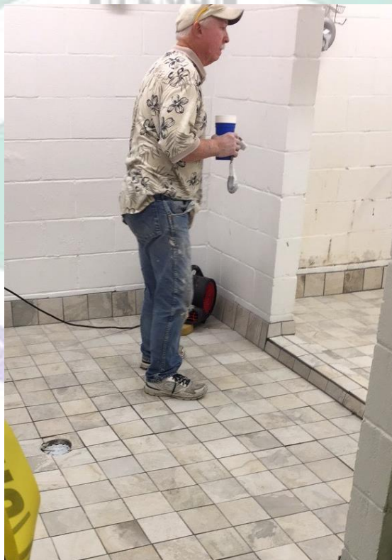
The shower room floor was tiled by Turner Tarrillion and his dad over the summer.
